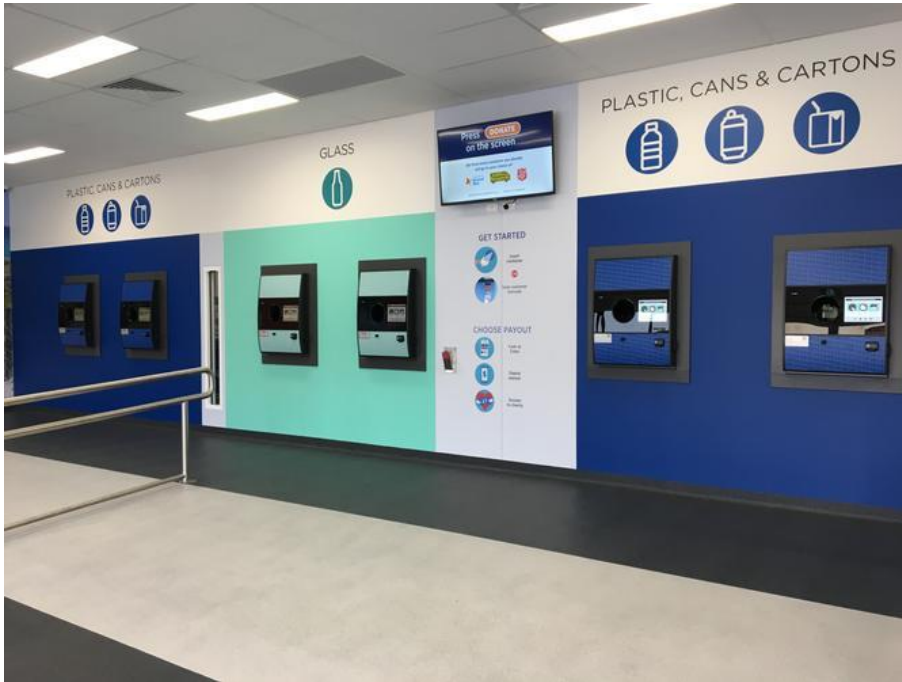
Figure 5: Small RVMs installed along wall, forming a mini recycling centre Credit: https://www.perthnow.com.au/community-news/stirling-times/was-containers-for-change-deposit-scheme-officially-up-and-running-c-1351180
